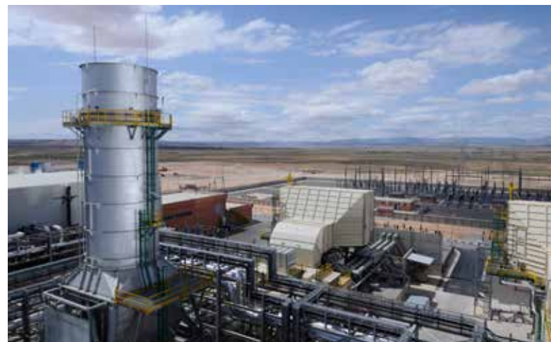
Thermo-solar power plant in Morocco (World Bank 2010)
