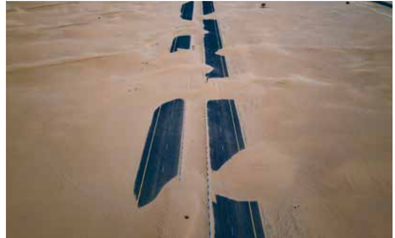
Road after a sandstorm in Dubai (Schwaerzler 2017).
